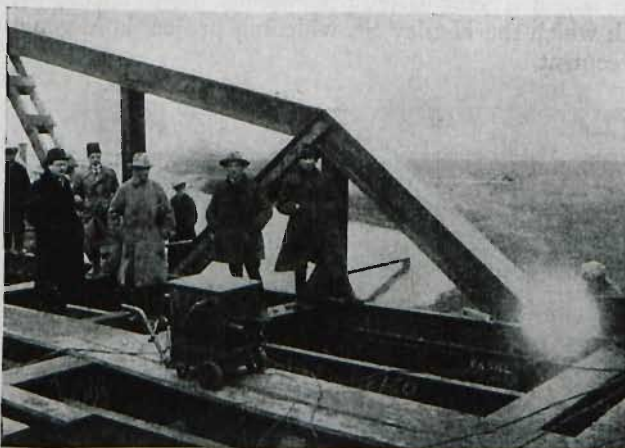
FIG. 2—WELDING AN END POST ON THE POLISH HIGHWAY BRIDGE Note the welding generator in the foreground.
