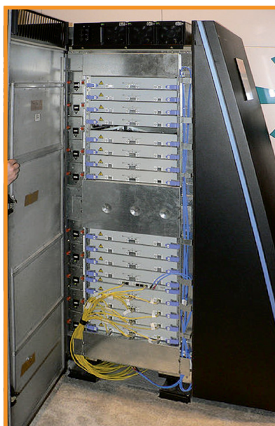
Fig. 4. One of computer cabinets
