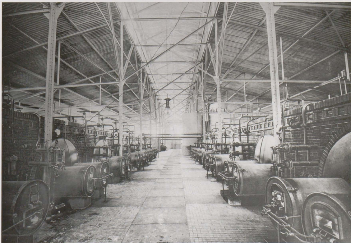
Boiler room, the Steaua Română Refinery – Câmpina, Prahova County
