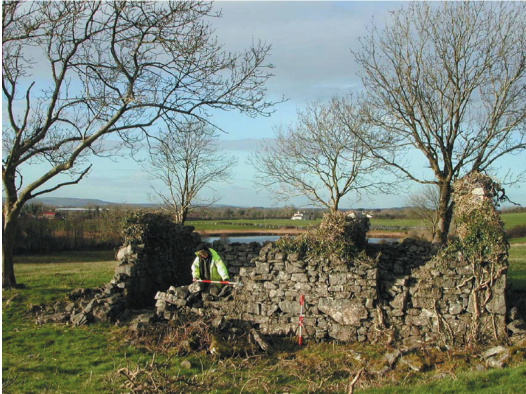
Recording early modern building remains on the N18 Ennis Bypass, County Clare (Aegis Archaeology Ltd)
