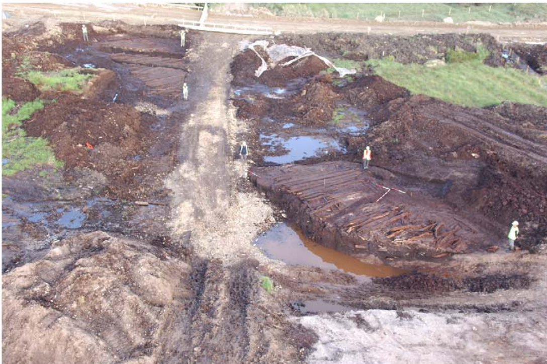
Plate 67: Aerial view of the causeway showing how the causeway dipped in the middle before rising towards the gravel island in the west. Looking east. (Photo: Hawkeye)
