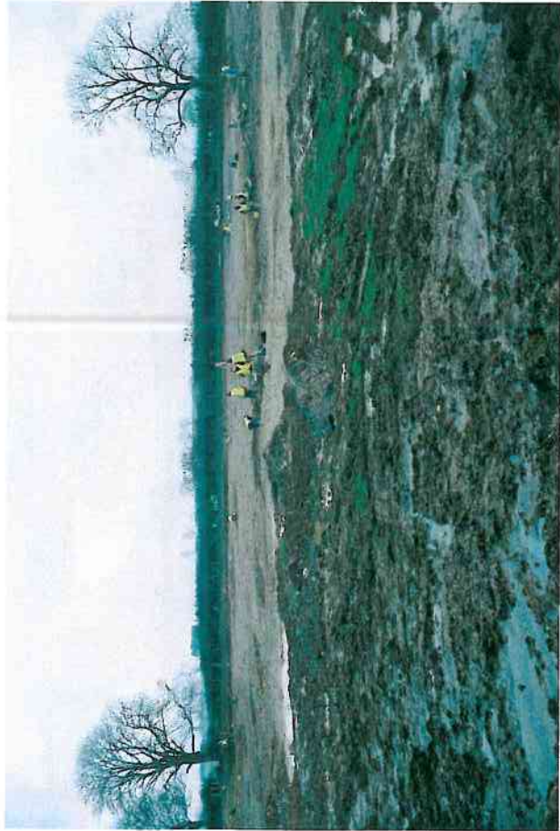
Plate 1: General view of ongoing work on the Lismore side of the townland boundary (Zones A and B), facing east (05_09_CP0024_05)
