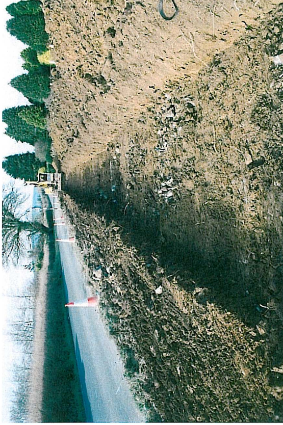
Plate 2: Stripping in progress at LA022:012 along eastern side of public road R435 (05_09_CP869_13)
