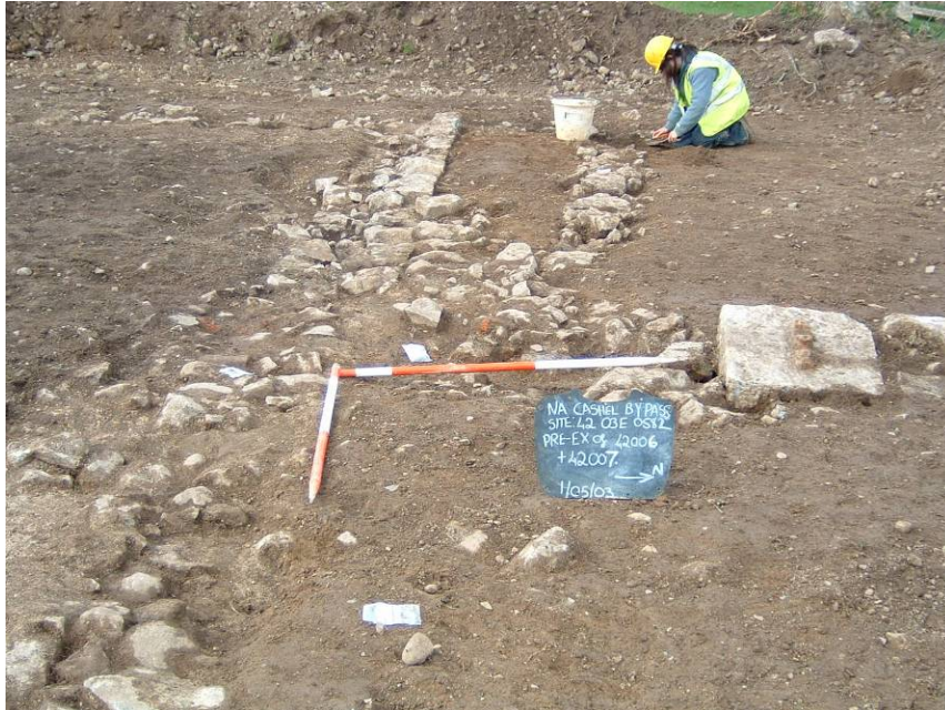
Plate 10: Pre-excavation of north-west corner of building, showing stone with iron insert (07) within fabric of path [17]. Looking south-west. Scales 1 m
